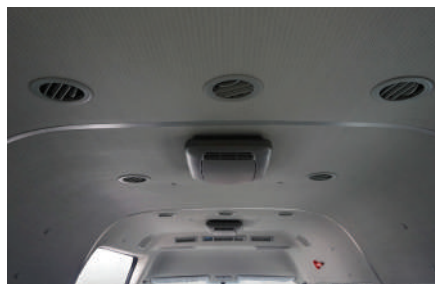
DOUBLE REAR A/C UNIT WITH 9 ROOF VENTS
